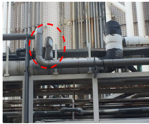
Nanya PCB 5 steam enter point
