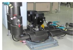
Hot Water Pump
