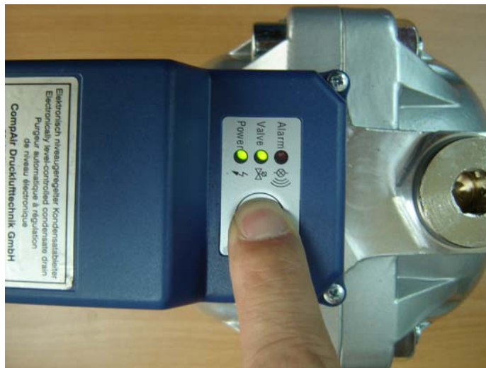
故障時：Alarm紅燈顯示(Red light Alarm)
