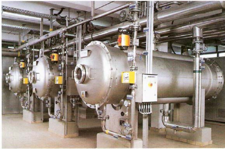
Rostock Water Works. Advanced Technology ozone generators (3 x 8.7 kg/h at 10 wt%)
