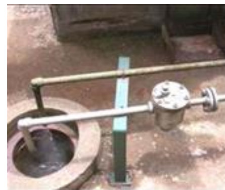
倒筒式祛水器排水洩漏
