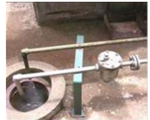
倒筒式祛水器排水洩漏
