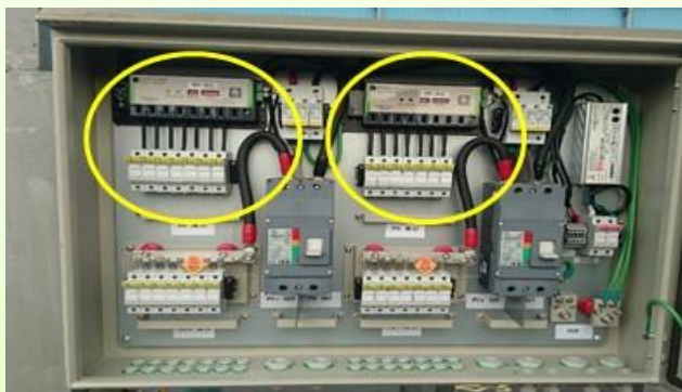
DC Panel-串接string meter
