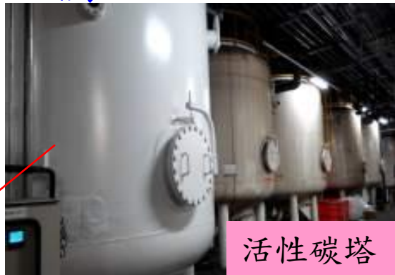
ACF(Activated Carbon Filter)
