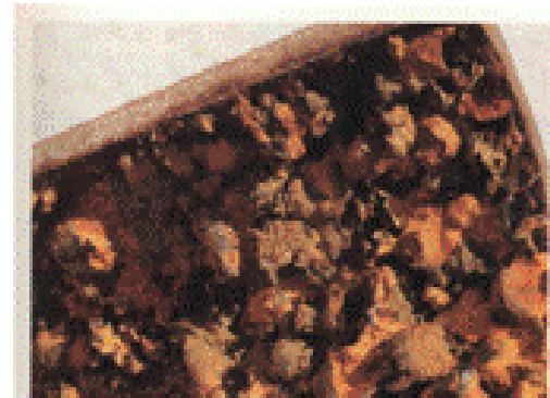
Figure 3.19 Small, hard tubercles on an essential service water system pipe in a nuclear reactor.
