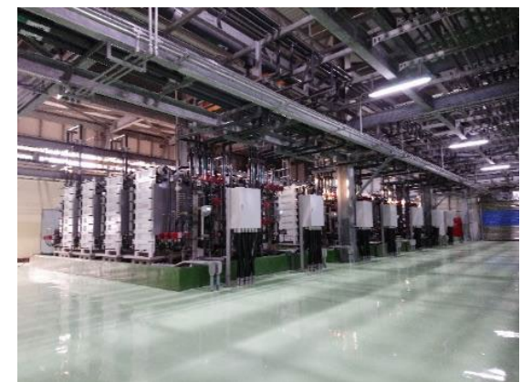
EDR Water Recycling System
