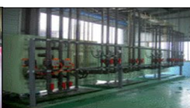
Recovery of wastewater from screw manufacturing factory for rinsing water by EDR process (450 m 3 /day)
