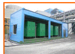
Recovery of wastewater from chemical company for cooling water by EDR process (800 m 3 /day)
