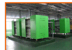
Recovery of wastewater from nylon fiber manufacturing company for cooling water by EDR process ( 800 m 3 /day)
