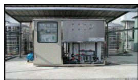
EDR desalination of Ground water for rinsing water ( 50 m 3 /day)
