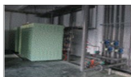
Recovery of wastewater from PCB manufacturing factory for cooling tower by EDR process (1200 m 3 /day)
