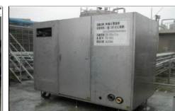
Desalination and reuse of RO concentrate stream (Food industry) (300 m 3 /day)
