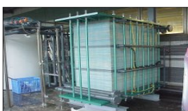
EDR desalination of RO reject for rinsing water (electronics) (300 m 3 /day)
