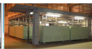
Recovery of fluoride-containing wastewater from wafer factory for scrubber by EDR process (1200 m 3 /day)
