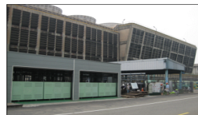
Desalination and reuse of direct cooling water from steel rolling by EDR process (China steel company, 550 m 3 /day)
