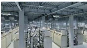
Cell stacks, Heat exchangers (2nd Floor)
