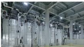
Tanks, Pumps, PCS (1st Floor)
